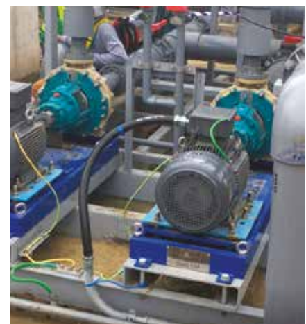
THAILAND, Electrochlorination plant Hypochlorite and seawater dosing pumps
